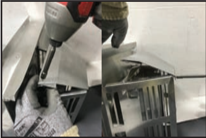
Figure 7.15 Wind Diverter Installed
